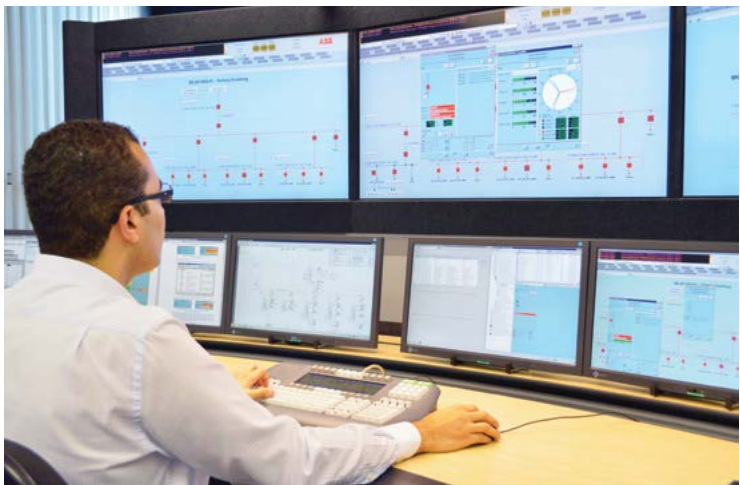
Energy Automation and Protection; Energy Scada, PRP, HSR, IEC 61850 Applications
